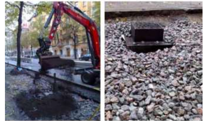
Creation of structural soil for trees in paved area. The pictures show structural skeleton with aerated bearing layer, an air inlet of type TLP 2333 Clarova with cover, addition of planting soil type D and aerated bearing layer around the air vent. (Photo: Örjan Isdahl).
