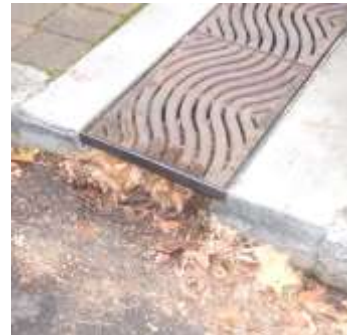
Clogged water access
